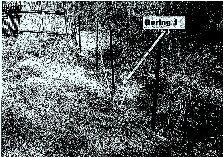
Photograph No. 1 : Failed embankment (looking Northwest) and approximate location of Boring No. 1.
